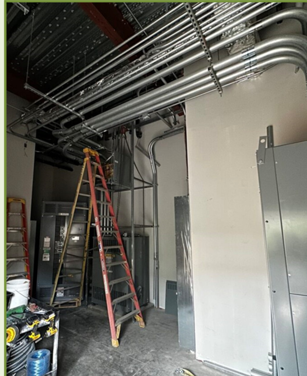
CENTRAL ELECTRICAL ROOM
