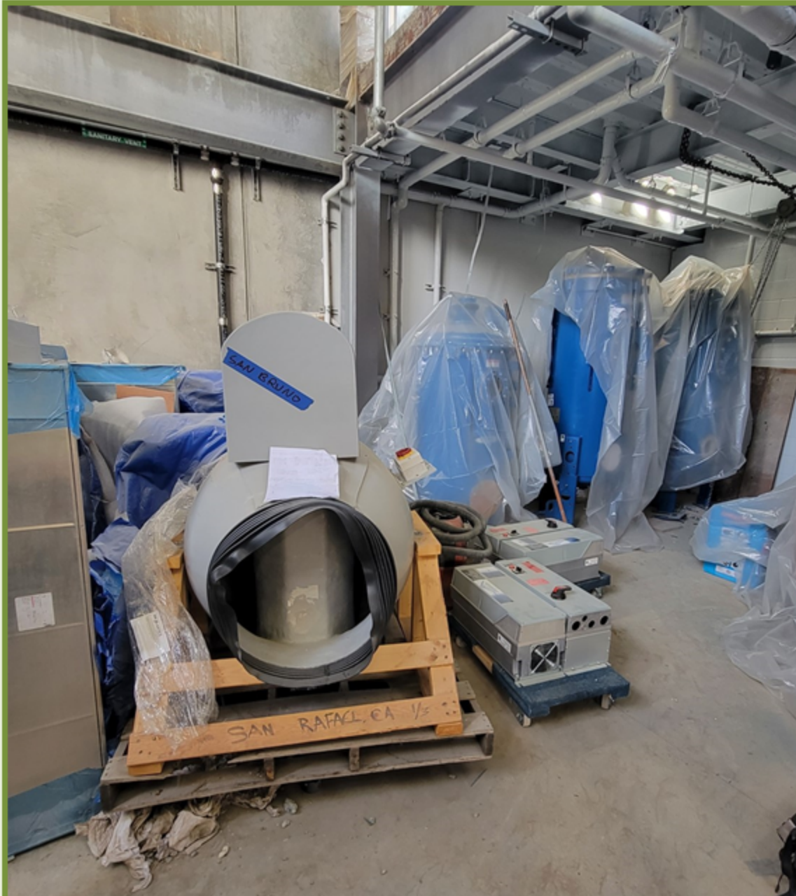
POOL PUMP ROOM
