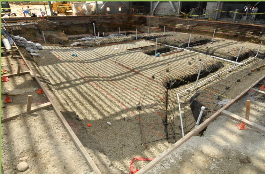
INDOOR POOL PLUMBING
