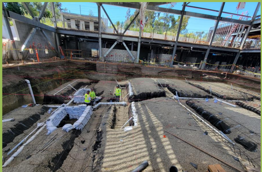
INDOOR POOL PLUMBING
