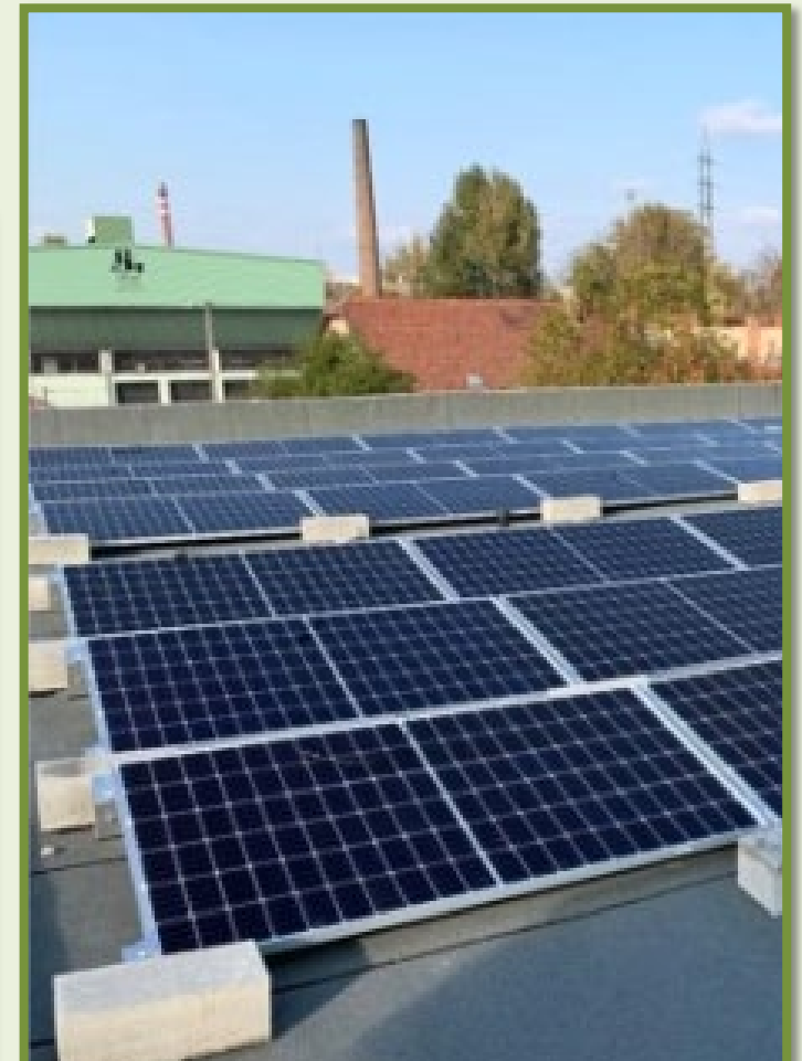
EXAMPLE OF BALLAST-MOUNTED SOLAR PANELS
