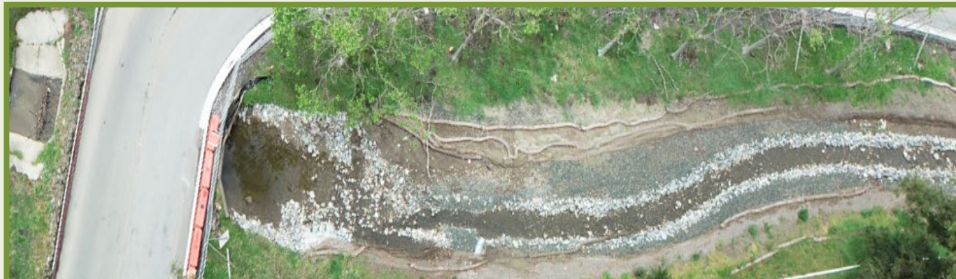
STORM DAMAGE - BANK EROSION
